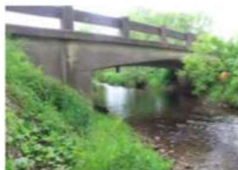
North deck drain and soffit delamination
