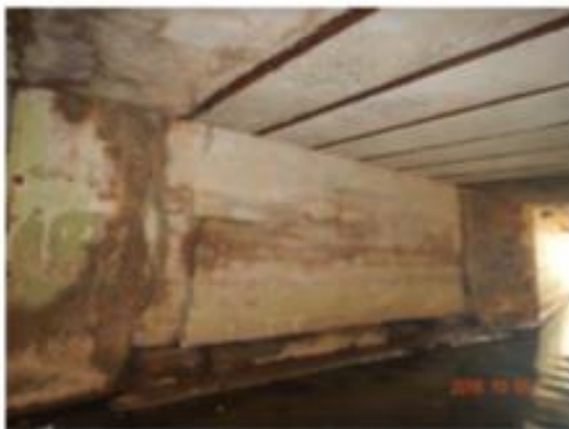
Image A.6 concrete culvert with a BCI of 48.0 (Poor)
