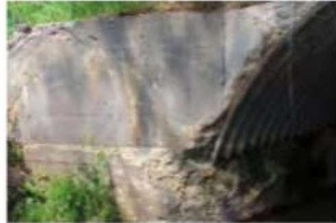
NW wingwall disintegration
