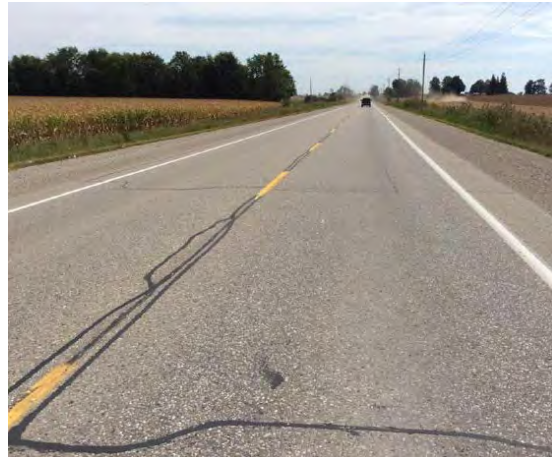
Image B.2. Rural Road with a PCI of 73.7 (Good)
