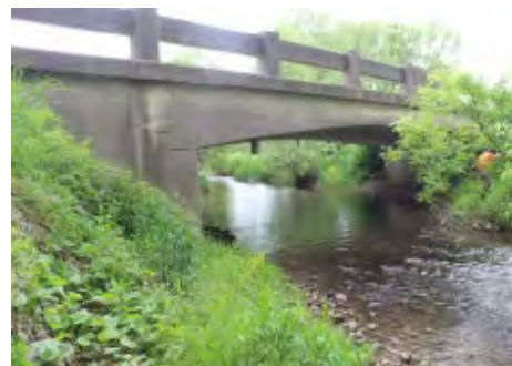
North deck drain and soffit delamination
