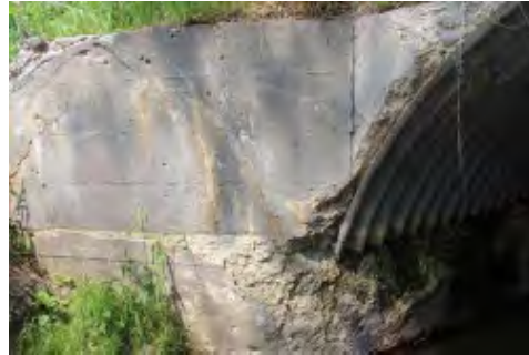
NW wingwall disintegration
